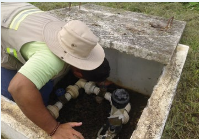
Inspection of the water chlorination system, part of Penonomé's support for community based organizations that supply water to local communities. Photograph courtesy of Penonomé.
