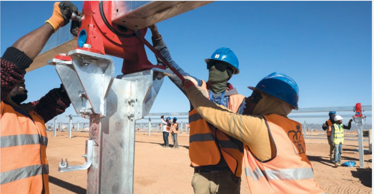
Construction workers at the Benban Solar Park in Egypt. Photograph by Dominic Chavez. IFC photo collection.
