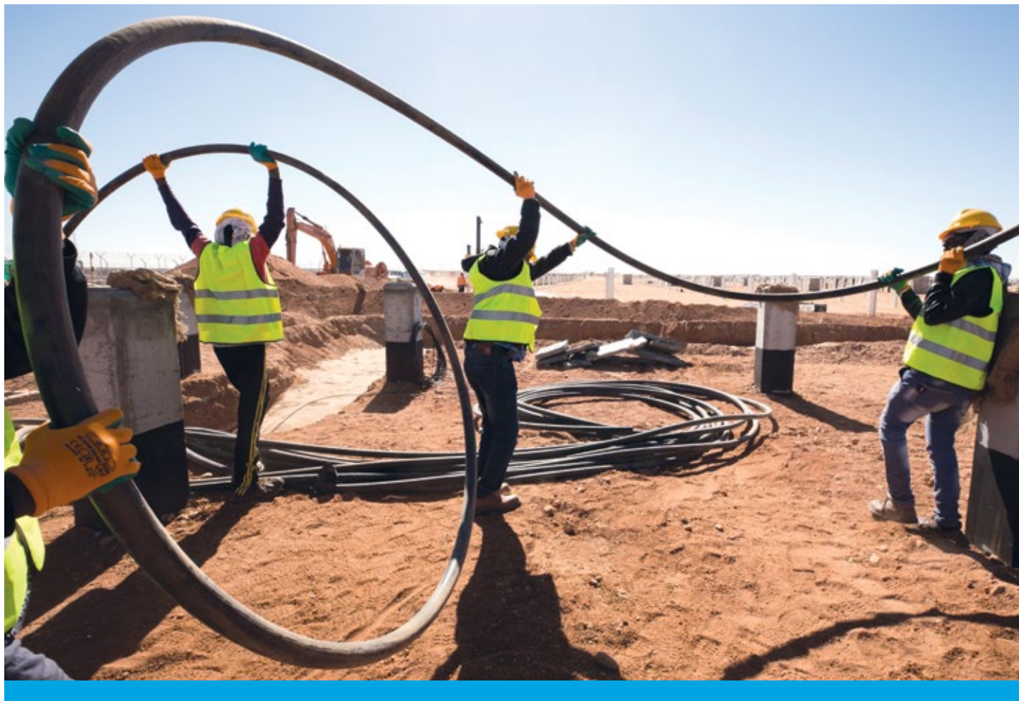
Workers carry medium-voltage cables at the Benban Solar Park in Egypt. Photograph by Dominic Chavez. IFC photo collection.
